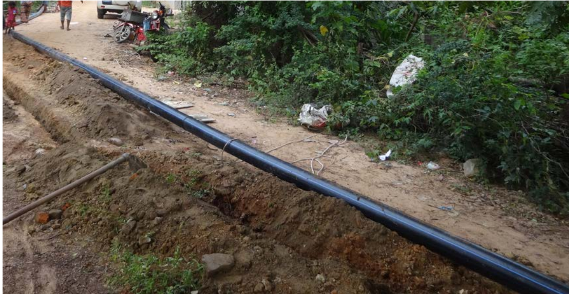
Above: W2016 Phon Sokun network, in Tbeng Khpos commune, Sammaki Meanchay district, Kompong Chhnang, 1 November 2017. Main water pipe and trench being dug – by hand - north of the village from the area of the railway. The contractor explained that he hired manual labour to excavate with hoes as this was cheaper.
