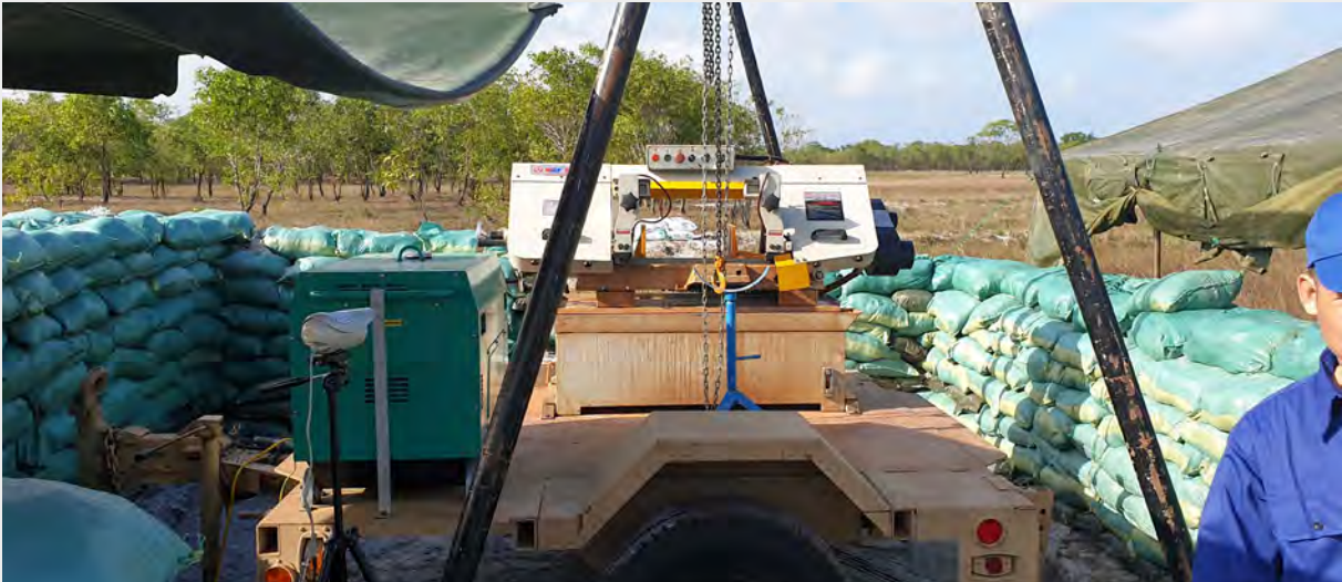
The mobile cutting system was set up in a sandbagged bunker area with the hoist and generator. The Wi-Fi camera system was very unreliable so another camera system with hardwire and LCD screen will be bought, as a replacement. This will be presented to VNMAC (estimated cost is US$ 200).
